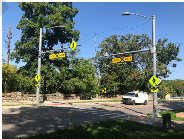
Figure 9 The crosswalk on Geddes Avenue at Gallup Path includes lighting at the crosswalk on both sides.
