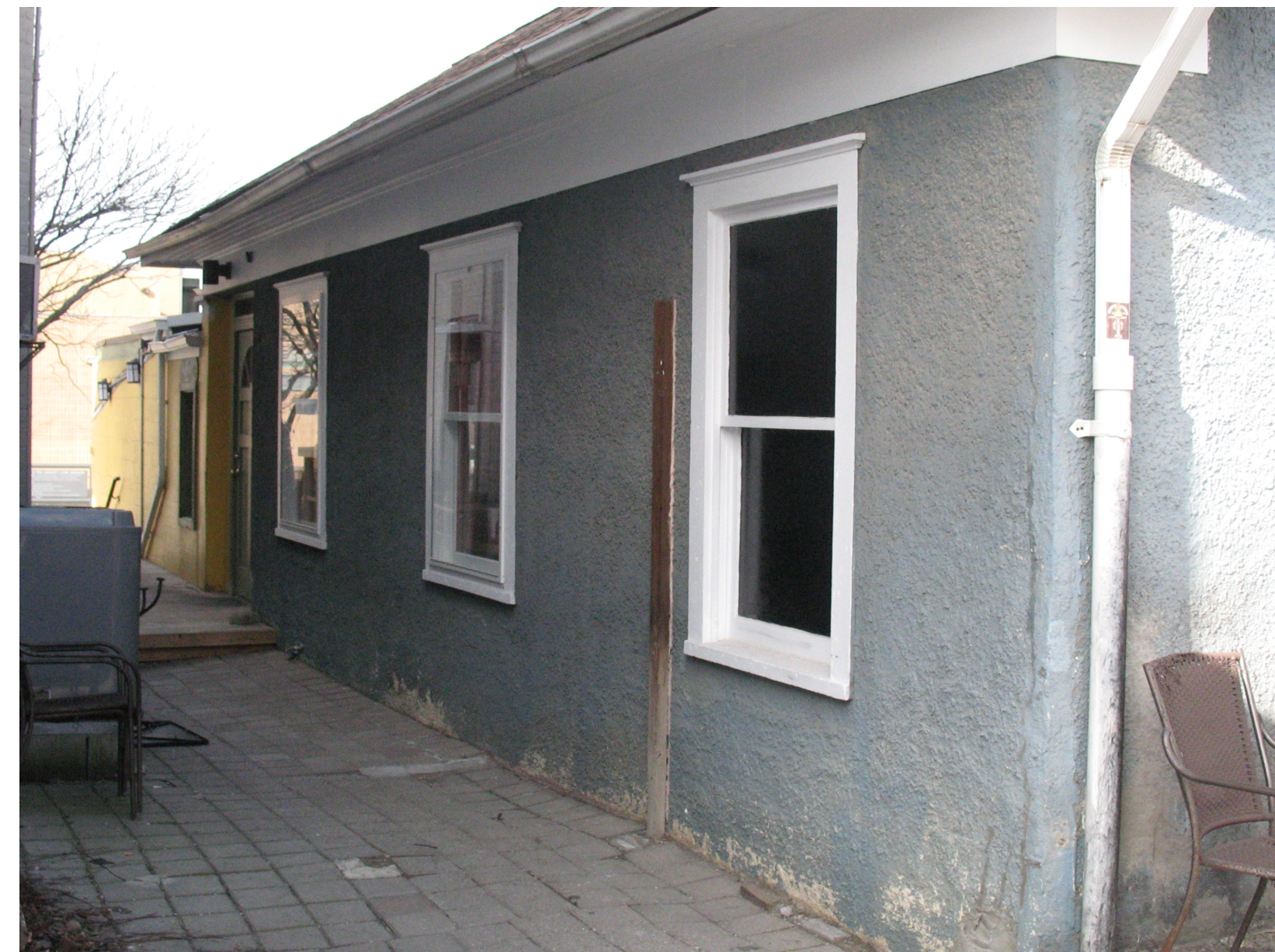
SOUTH ELEVATION FROM EAST. NOTE COMMERCIAL ADDITION AT LEFT OF ORIGINAL STRUCTURE
